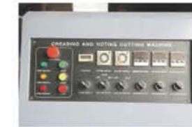
Electric box (front)
